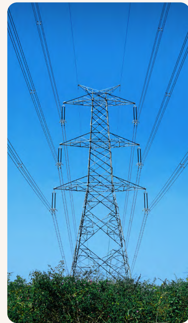
Transmission line – AXIA Collection
